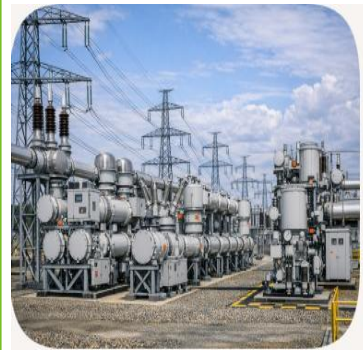
Figure 5: 400KV GIS Outdoor Configuration
