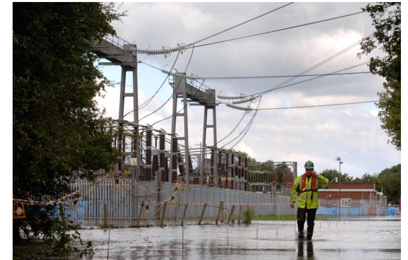
Flooded UK substation
